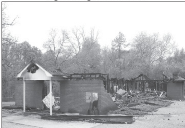
Larissa C.M.E. Church destroyed by fire
